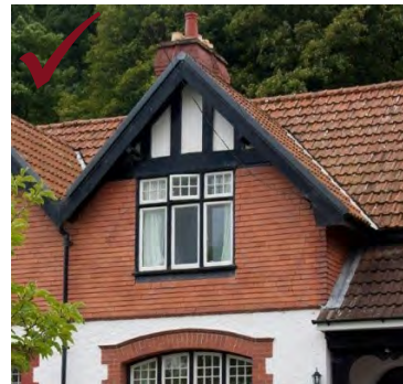
Above: traditional tile hanging and mock timbers to upper storey of former coastguard house
