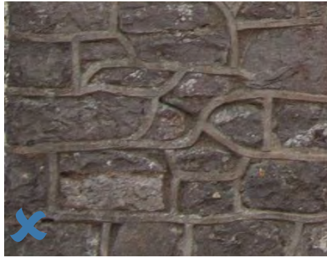
Inappropriate pointing to stone wall
