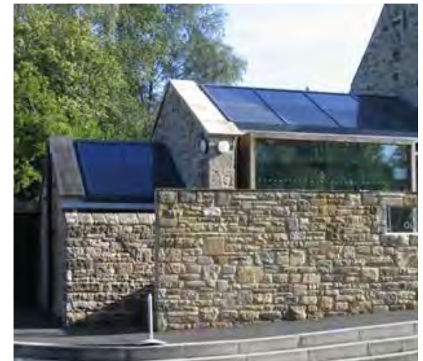
Above: PV installation integral to building design
